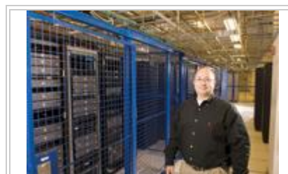
BlueBridge Networks CEO Neil Adelman in the secured computer area that houses clients' data.
